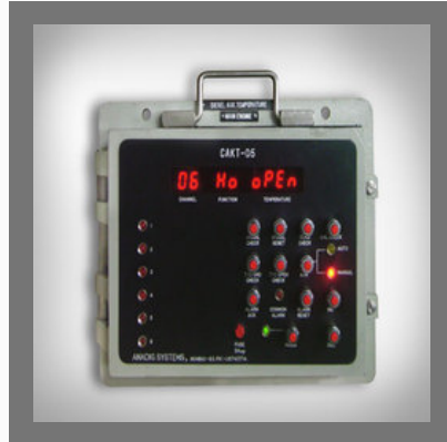
Temperature Monitoring System
